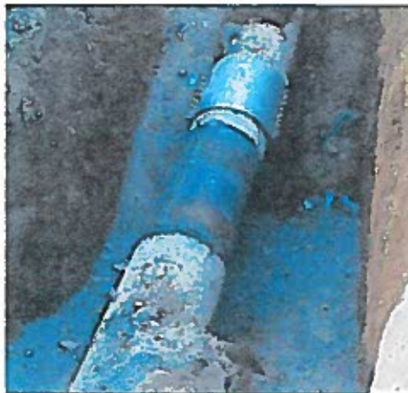
Photo of patch applied to a minor blow out that occurred last June.
