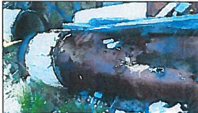
Photo of blow out last June
